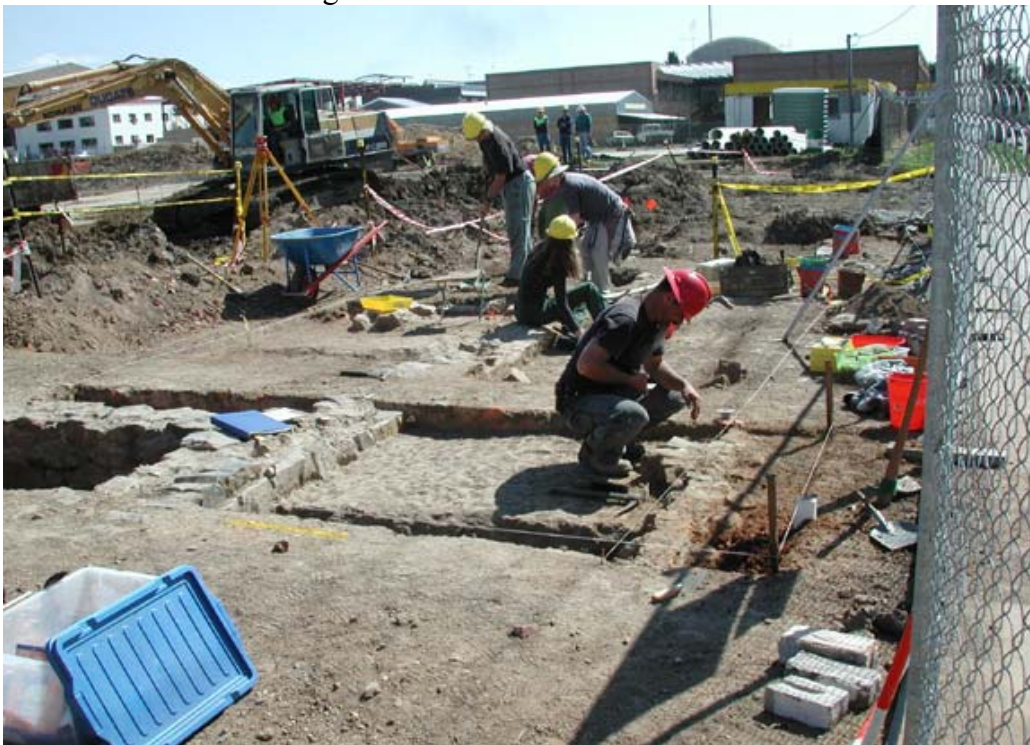
McLean's Corner, Armidale: archaeological excavation of the house frontage proceeding side by side with the demolition work for the development
