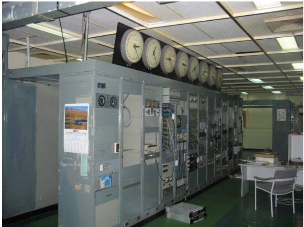
The Control Panel of the Area A VLF Facility
